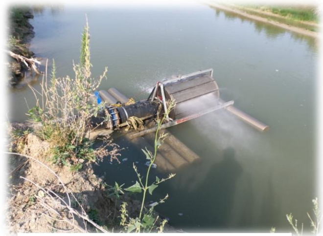
Figure 7. Screened drum on floating pump.
