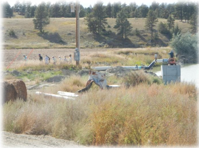
Figure 4. Power pole at reconstructed pump site. Photo credit: Karin Boyd.
